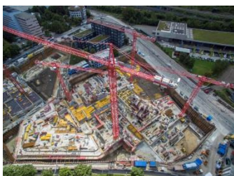
Four WOLFF cranes, commissioned by Porr Deutschland GmbH, are currently working on the Blue Tower and the White Tower at the Bogenhausener Tor.
