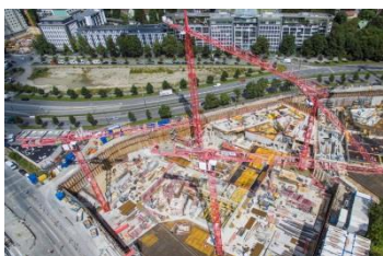
Thanks to the precisely coordinated jib radii and tower heights, the WOLFF top-slewing cranes can slew underneath each other without a problem, despite the confined conditions of the construction site.
